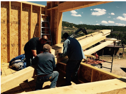
Hauling those heavy beams into the upstairs space from the "dock" seen in the photo at right.
