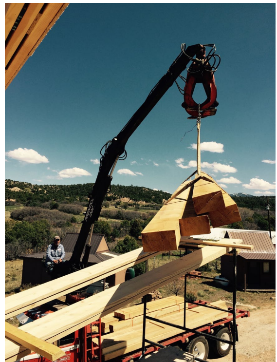
A batch of beams is hoisted up to be brought in through the south-facing window opening of what will become a second floor bedroom
